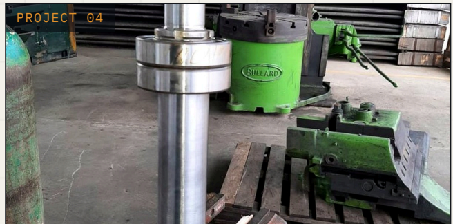
PROJECT 04 ROTATING EQUIPMENT PetroCedeño Upgrader, S.A. Pump and motor repair Jose Industrial Complex, Anzoátegui
